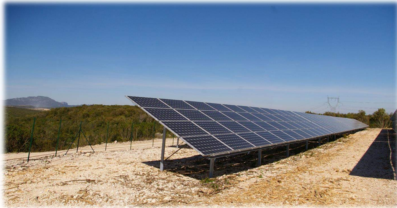
Champs photovoltaïque du Murles (D.Delat)
